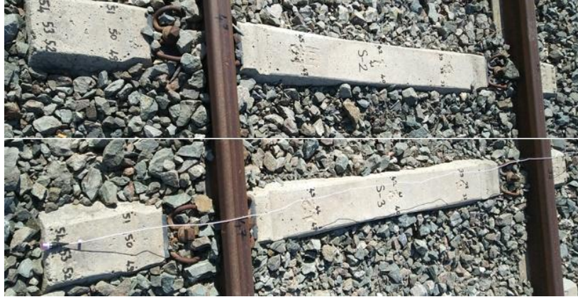
Figure 5. No visible cracks observed concrete railway sleeper samples (S-1) in the field
